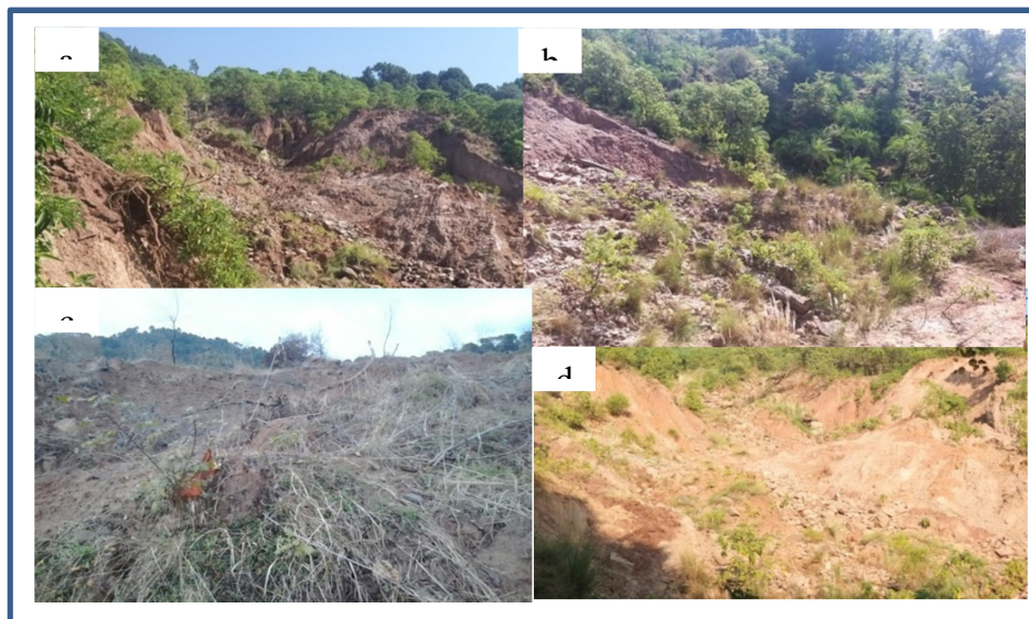
Fig. 3. Shows lithological characteristics of the slide zone: a) The area on the left of the slide zone, which was exposed due to the activity in the region; b) shows the presence of weathered rock material from the scarp region; c) the central part of the slide zones in the western side indicating weathered soil with uprooted trees and bushes, d) uneven topography on the southeast part of the slide in the slide zone with sandy to fine soil particles.
